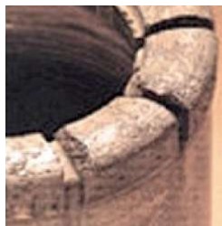
LOSS OF INSIDE DIAMETER
